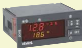
Controller on cold-water generator
